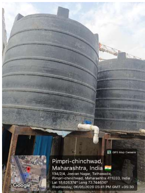
Drinking water Facility for labour
